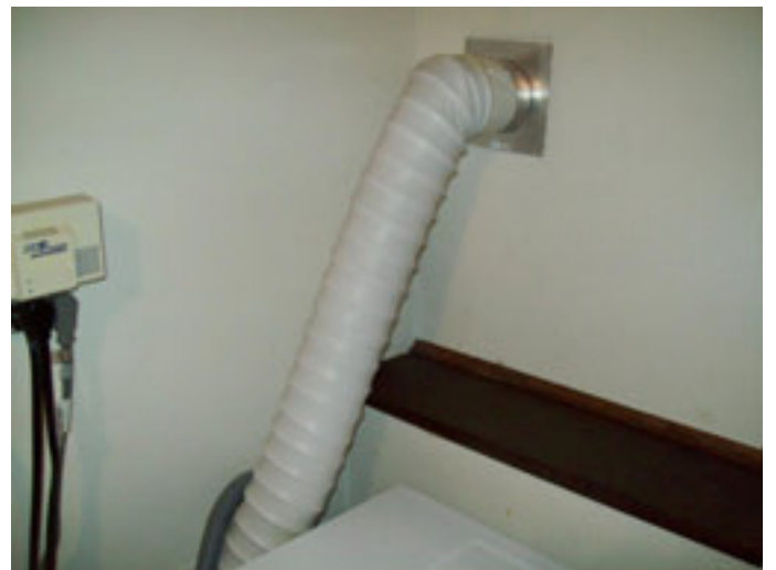
Dryer vents through improper material
