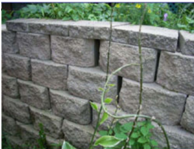
Shifting in rear retaining wall
