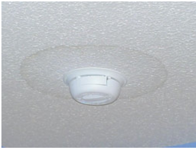
Ceiling stain, upper hallway - dry
