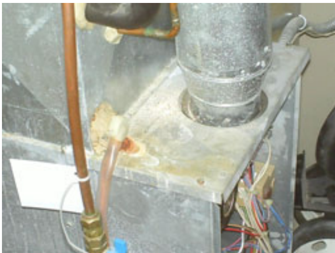
Rust / debris from vent pipe
