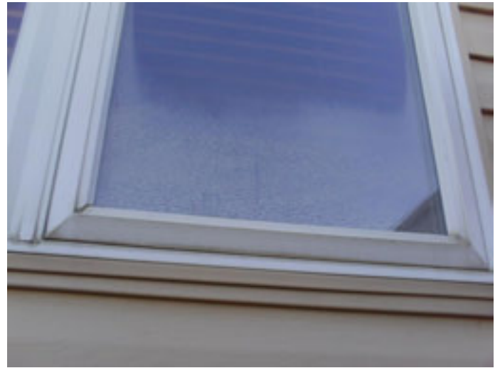
Moisture between window panes
