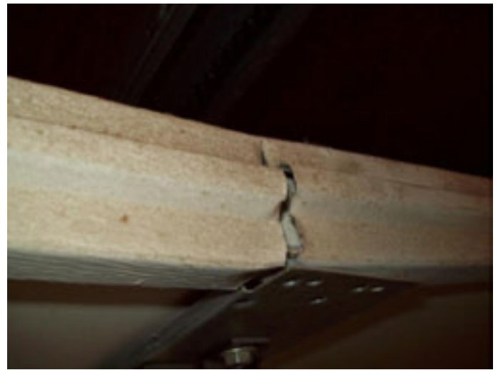
Top garage door panel cracked
