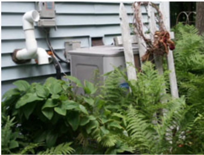
Improper clearance around A/C unit
