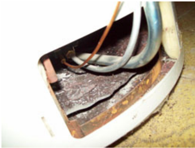
Rust flakes in chamber
