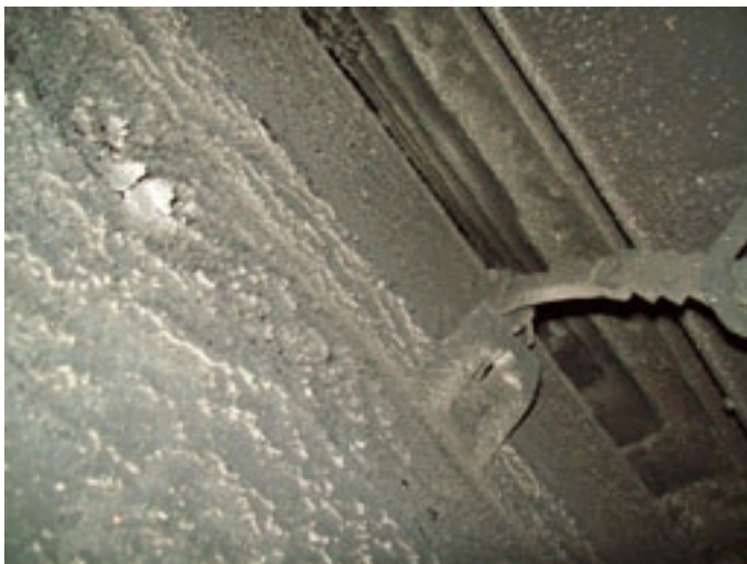
Creosote build up, main fireplace
