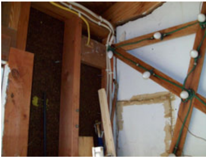
electrical wires subject to damage, (garage)
